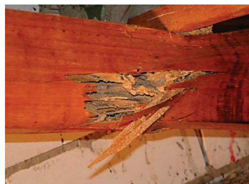
Termite damaged wood in the roof of a house. You can avoid this happening to you.
