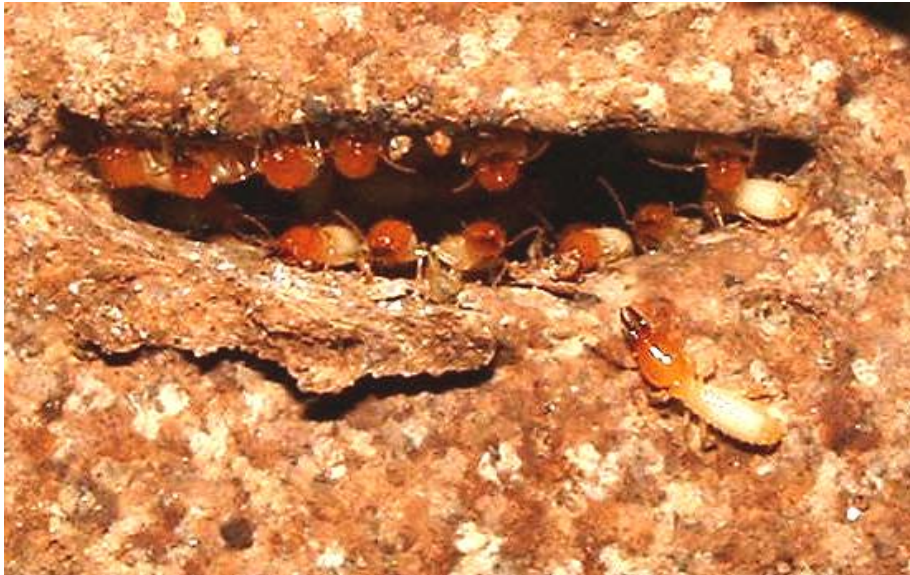
A group of Coptotermes soldiers vigilantly defending their entry point in a besser block wall after the plaster was removed to expose them.
